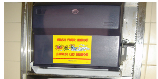
Removed accessible tri-fold dispenser w/ inaccessible fixture
